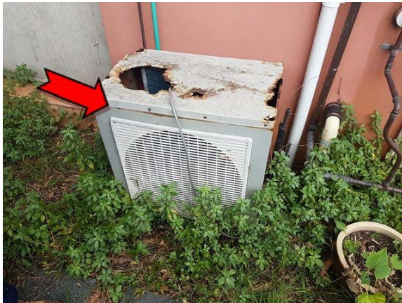
Photo 9. Exterior, south-west elevation, air conditioning unit – suspected ODS-containing unknown refrigerant.
