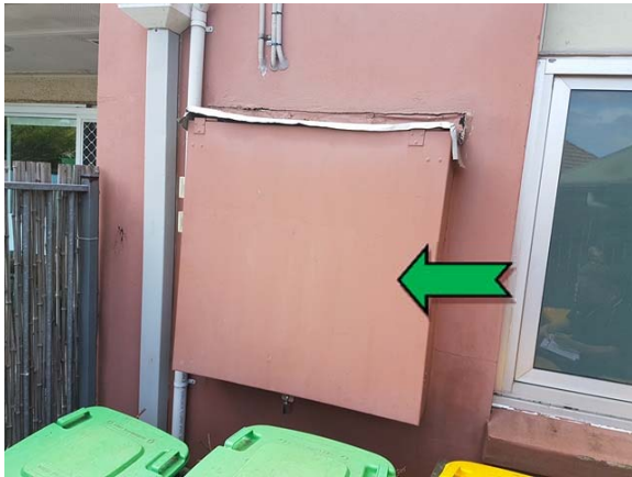
Photo 3. Exterior, south-east elevation, electrical backing board – suspected non asbestos-containing bituminous backing board.
