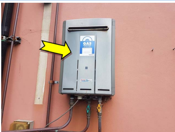
Photo 5. Exterior, south-west elevation, hot water heater – suspected SMF internal insulation material.
