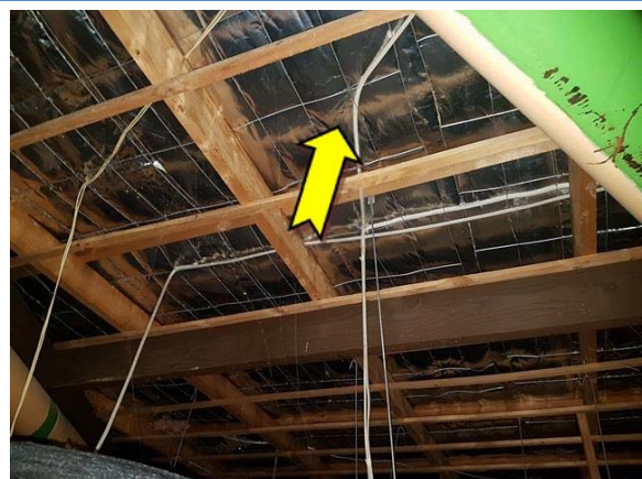
Photo 6. Interior, ceiling space, throughout – suspected SMF sarking insulation material.
