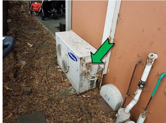
Photo 8. Exterior, south-west elevation, air conditioning unit – R410A non ODS-containing refrigerant gas.
