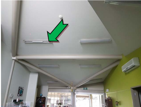
Photo 7. Interior, throughout, double tube fluorescent light fitting – suspected non PCB-containing capacitors.
